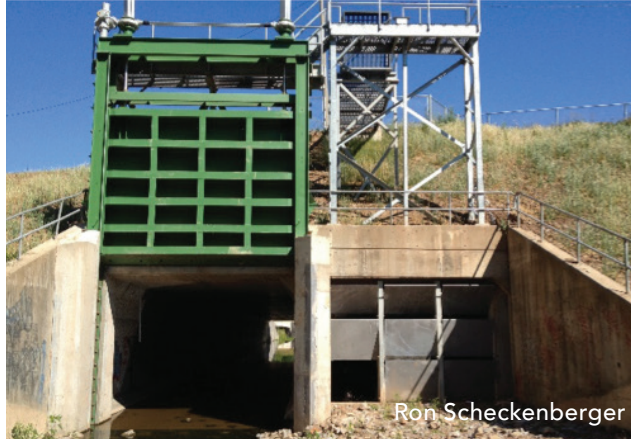
Twin cell culvert system, Davis Creek, City of Hamilton, Ontario. Left cell is to be fitted with an automated flood gate; right cell is fitted with a back-up manual gate.
